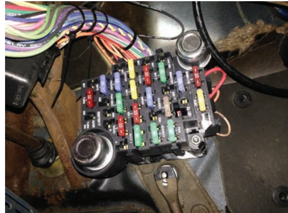
Fuse Block mounted under Dash in 1974 Duster
